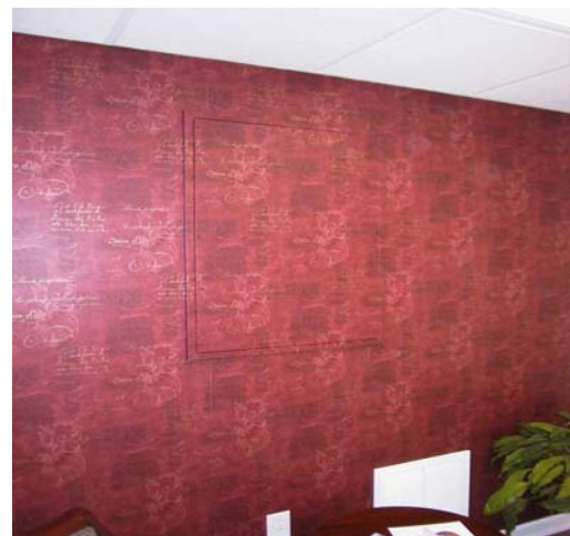
Close-up of Access Panel
